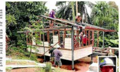
Sharing in caring: The team of 20 volunteers working hard to build the new house for Baid (left) and Ima.
